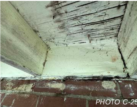
PHOTO C-25 Porch Sheathing and Framing Water Damage
