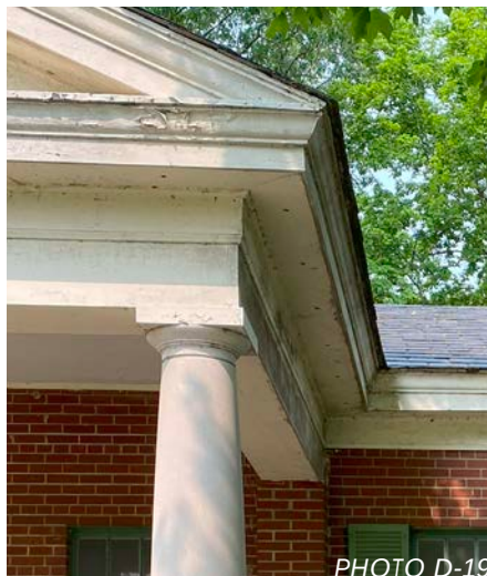
Column Capitol Detail Photo. This Photo showing typical paint deterioration.
