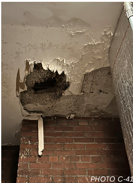
Damage to Ceiling in HVAC Room
