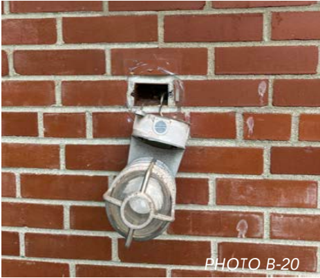
PHOTO B-20 Security Light Fixture hanging off of the wall.
