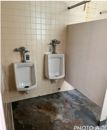
PHOTO A-30 Bathroom Conditions
