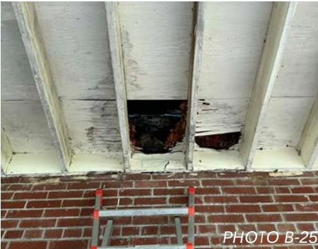
PHOTO B-25 Porch Sheathing and Framing Water Damage
