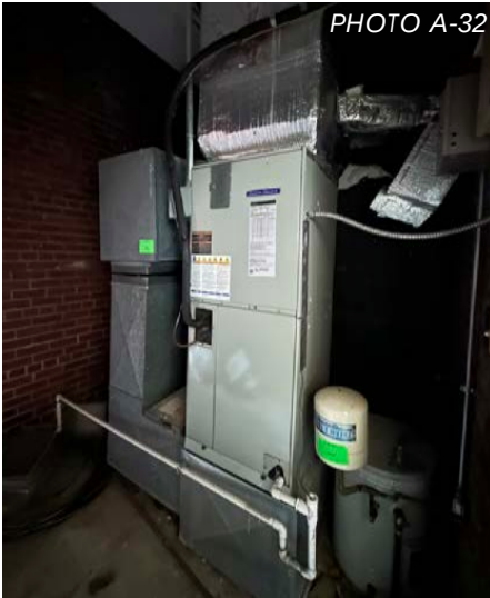
Existing HVAC System
