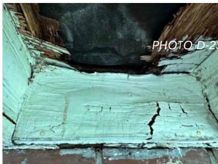
PHOTO D-23 Damaged Frieze Board and Sheathing
