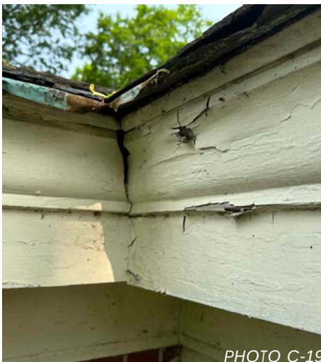
Typical Gutter/Frieze Board Detail. This Photo showing typical paint deterioration.
