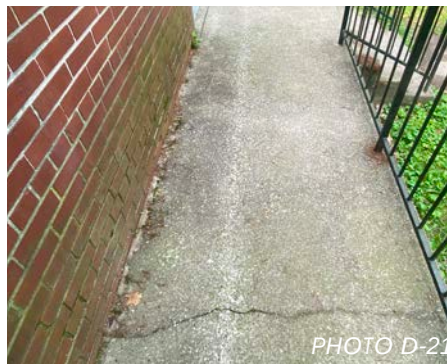
Photo of crack in concrete stoop.
