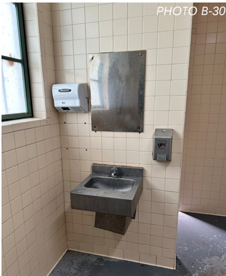
PHOTO B-30 Bathroom Conditions
