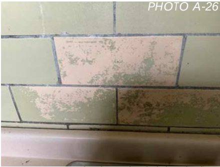
PHOTO A-26 Damaged Glazed Brick in Kitchen
