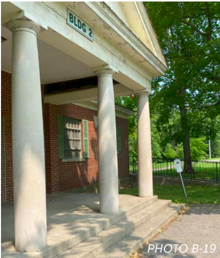
Concrete Columns Note missing frieze board
