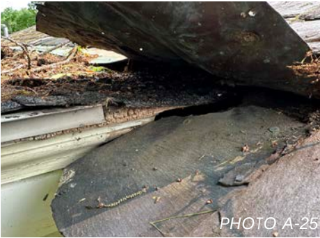
PHOTO A-25 Porch Roof Flashing Failure Detail
