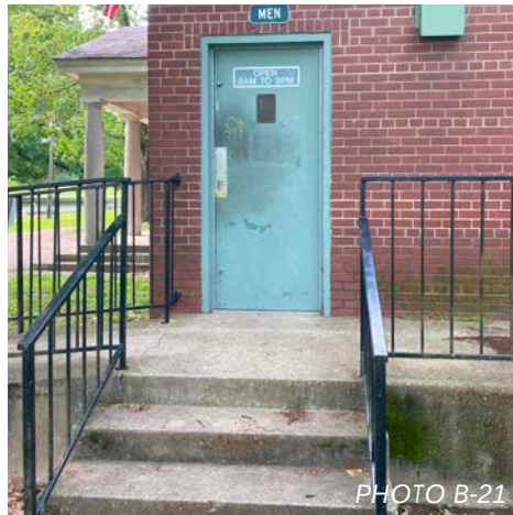
Photo of Men's Restroom Door, Steps and Railing.
