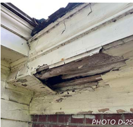
PHOTO D-25 Porch roof/Pitched Roof Cornice deterioration Photo
